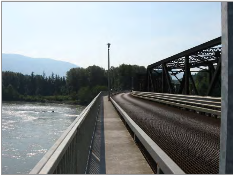
Figure 12. Old Skeena Bridge. Cyclists are not allowed on the deck.
