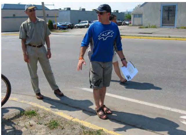
Bruce Martindale points out the lip on the gutter pan in the bike lane on Sparks St.
