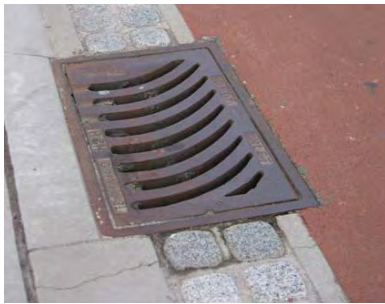
Bike friendly drainage grate example Photo: H.Redman
