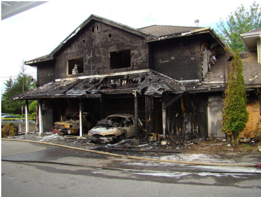
Townhouse complex fire that displaced 50 people for several days.
