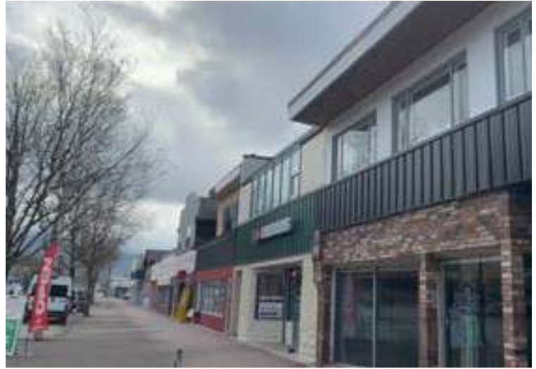
Above: In 2023, through a contractor, the City of Terrace removed the dilapidated canopy (shown at left) from the 4600 block of Lakelse Avenue. Businesses continued to work on facade improvements (shown at right) into 2024. More information is also available in the Development Services section of this report.
