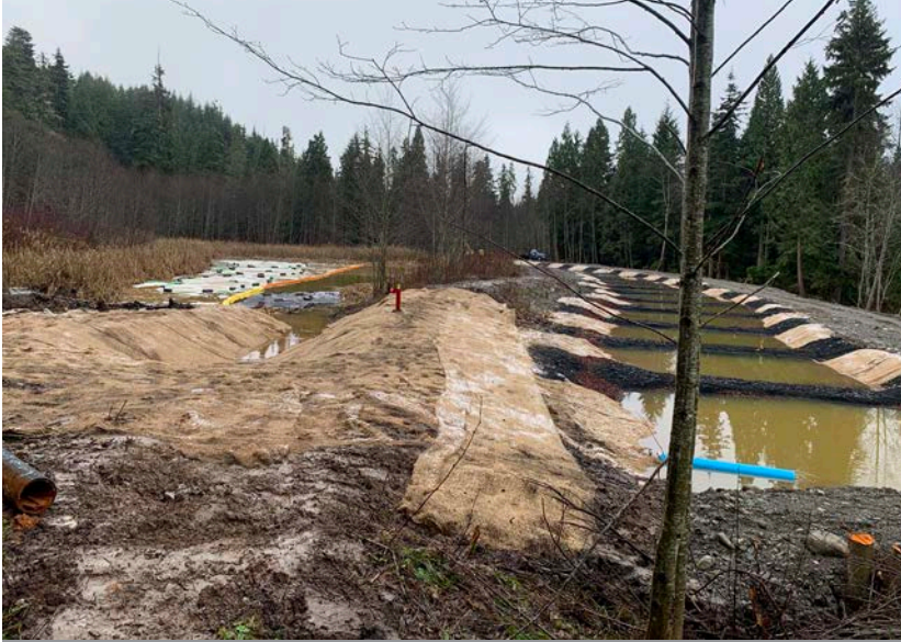
Above: In 2021, Public Works constructed an approximately 1 km long powerline and leachate treatment system and continued ground water quality monitoring at the City's closed landfill. They also undertook several environmental studies and updated the closure plan. Staff took on a significant portion of this work, resulting in substantial cost savings.
