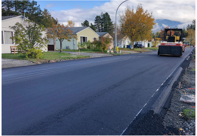
Above: In 2021, Public Works crews completed road reconstruction on Weber Ave. and replaced aging water and storm mains.
