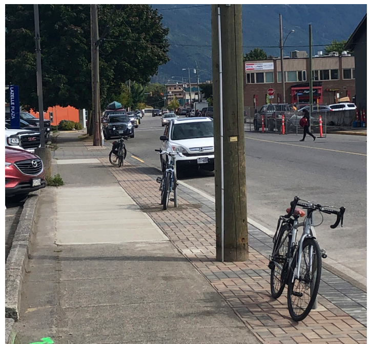
Above: In 2021, Public Works designed and oversaw construction of the Lazelle Boulevard Enhancement Project, Phase 1. Phase 2 is planned for 2022.
